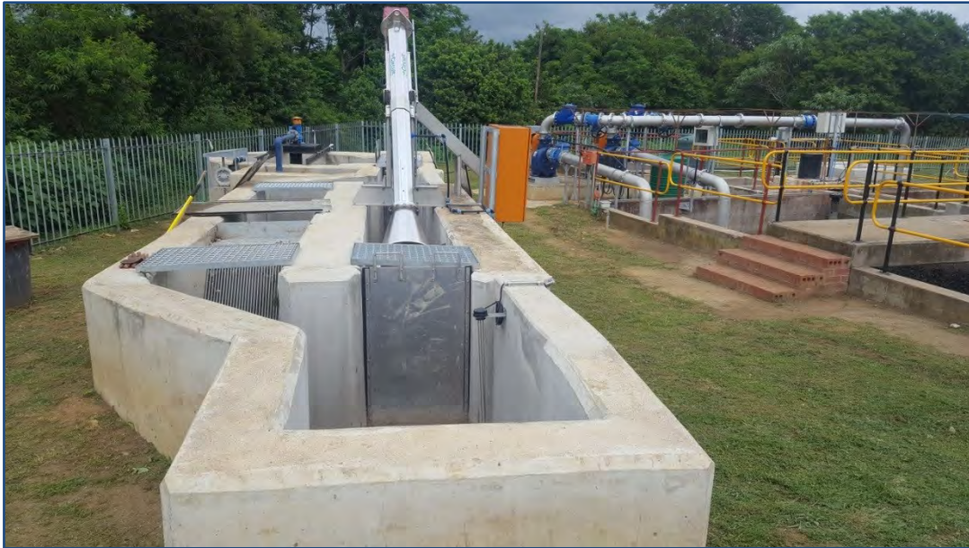
Figure 19.39 Lynnfield Park WWW head of works showing manual and mechanical screening channels.
