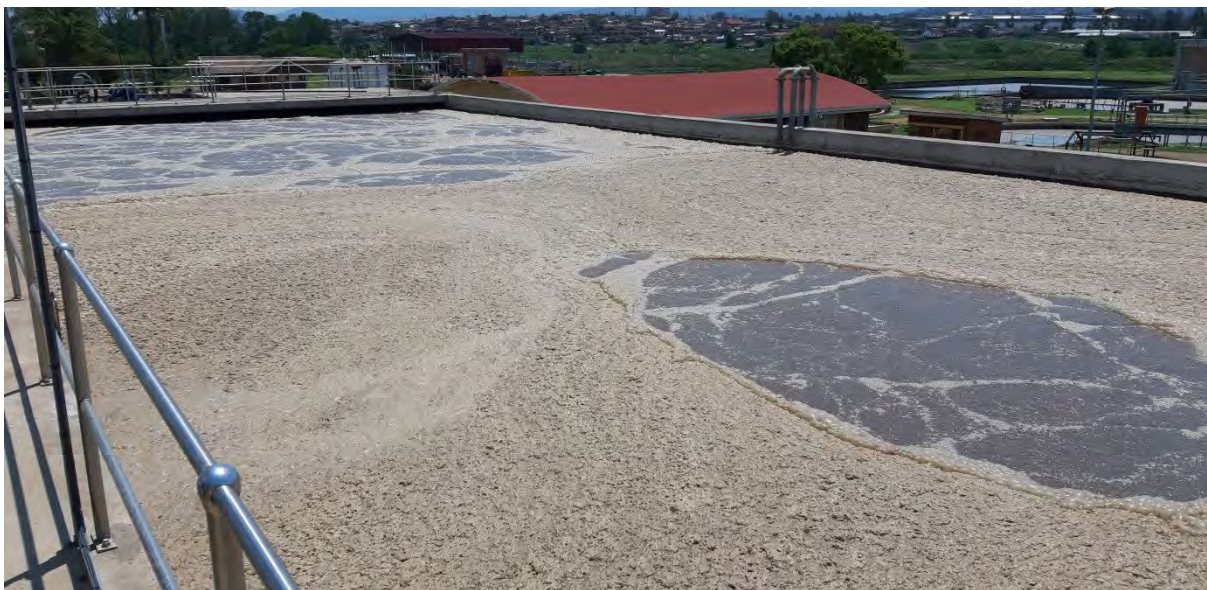
Figure 19.4 Darvill Aeration Basin.
