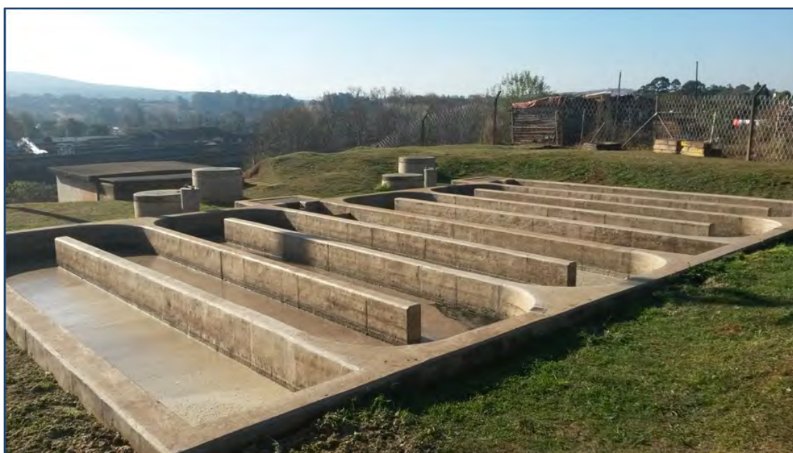
Figure 19.29 Howick WWW Chlorine Contact Tank.
