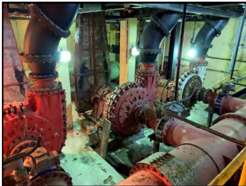
Figure 19.27 Alkantstrand B-Line pump sets (not operational) (Mhlathuze Water 2022: 53).
