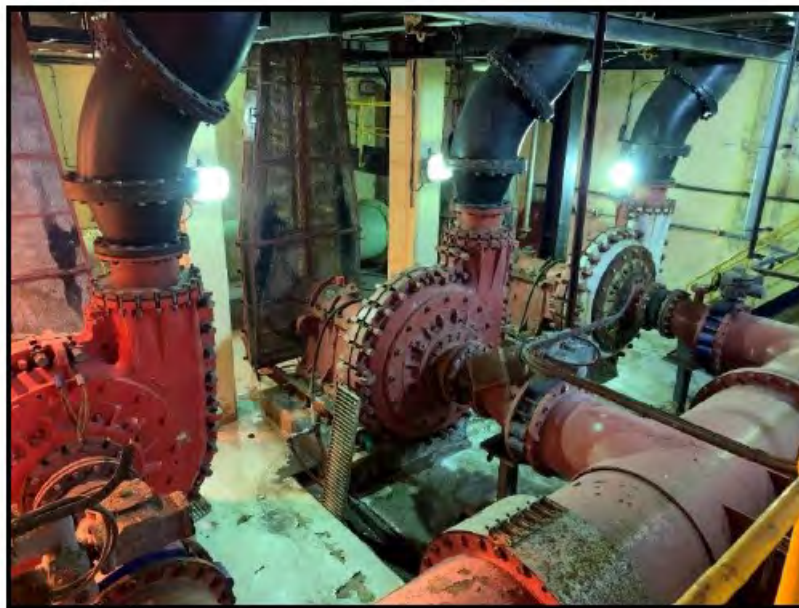
Figure 19.27 Alkantstrand B-Line pump sets (not operational) (Mhlathuze Water 2022: 53).
