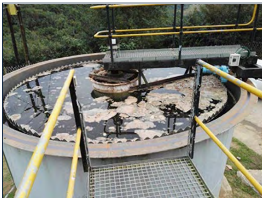
Figure 19.67 Camperdown Clarifier No. 2.
