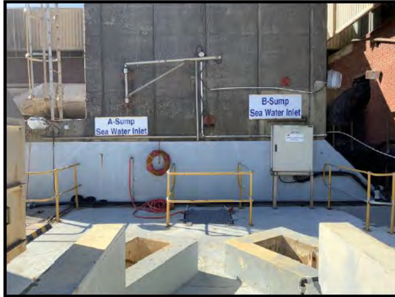
Figure 19.26 Alkantstrand seawater dilution infrastructure (Mhlathuze Water 2022: 53).
