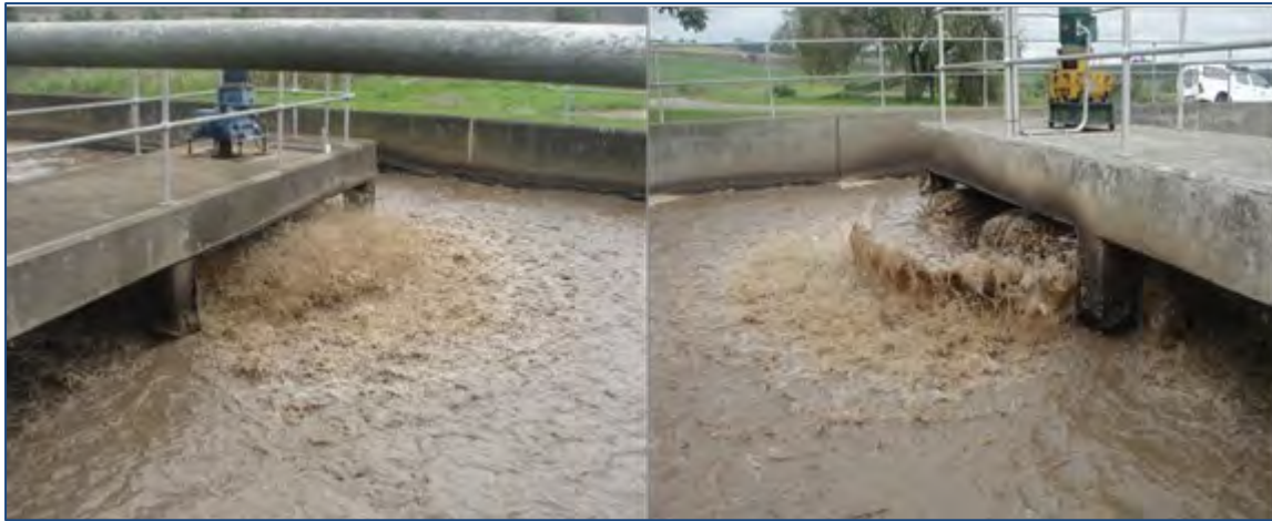
Figure 19.59 Different Mechanical Surface Aerators in Cool Air Reactor 1 and 2.
