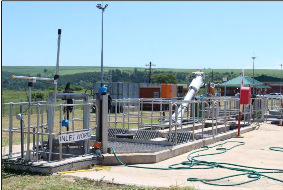
Figure 19.79 Head of Works Trust Feeds WWW.
