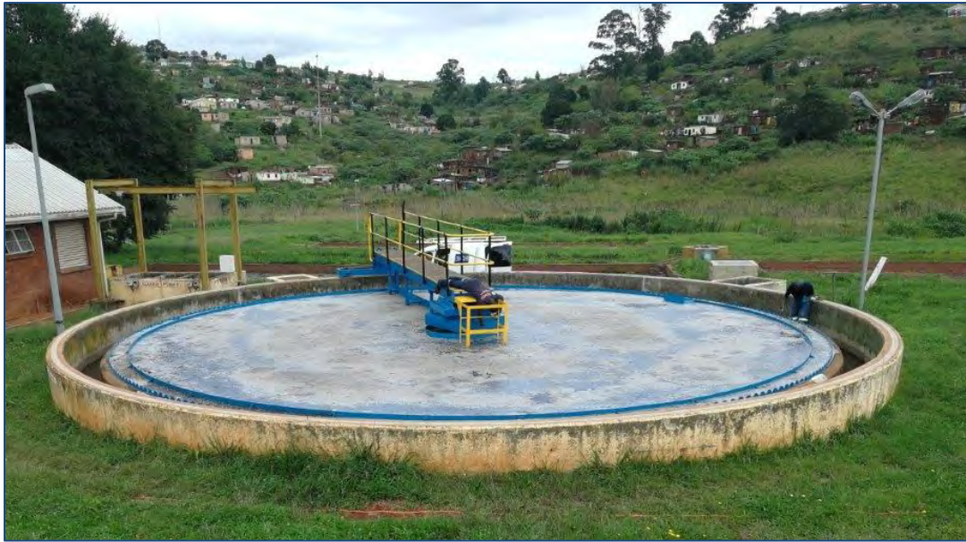
Figure 19.12 Clarifier No. 1 Ixopo WWW.
