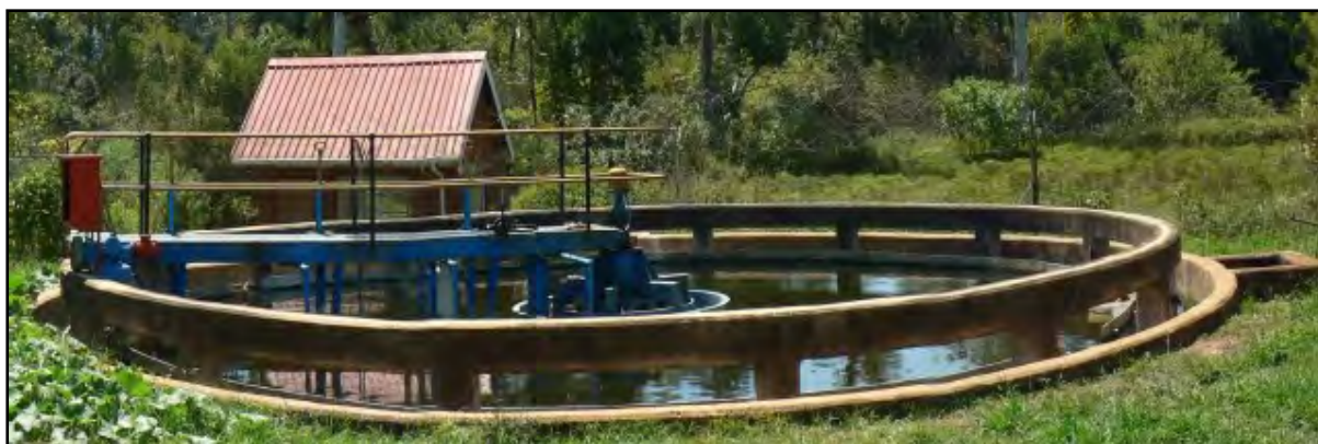
Figure 19.73 Richmond WWW clarifier.
