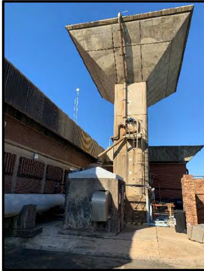
Figure 19.25 Surge tower (Mhlathuze Water 2022: 22).
