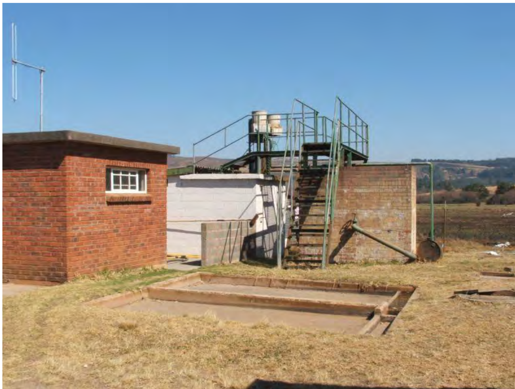
Figure 7.76 Lidgetton WTP sand wash bays with old dosing system (uMgungundlovu District Municipality 2010)
