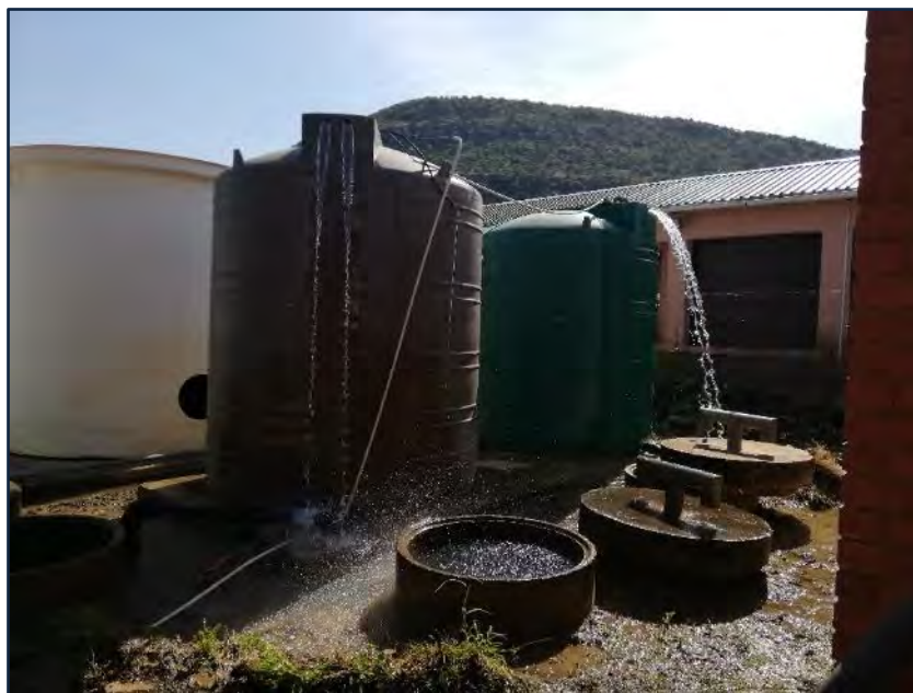
Figure 13.31 Tugela Estates WTP reservoirs (Umgeni Water 2019).
