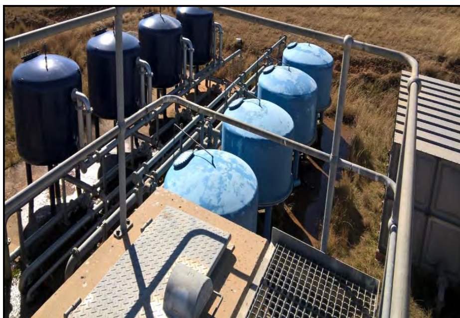
Figure 13.47 Zwelisha Moyeni WTP (Umgeni Water 2017)
