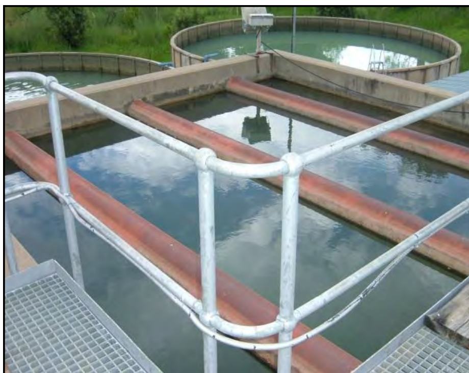
Figure 13.53 Colenso WTP (Umgeni Water 2017)
