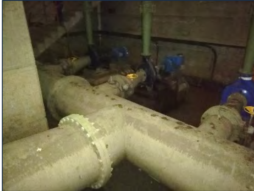
Figure 13.39 Olifantskop raw water pumps (Umgeni Water 2019).
