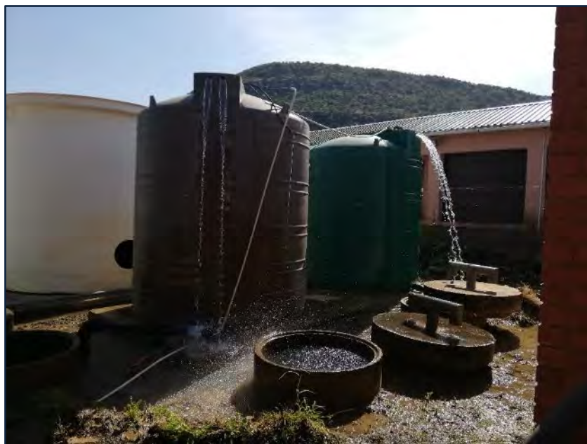
Figure 13.31 Tugela Estates WTP reservoirs (Umgeni Water 2019).
