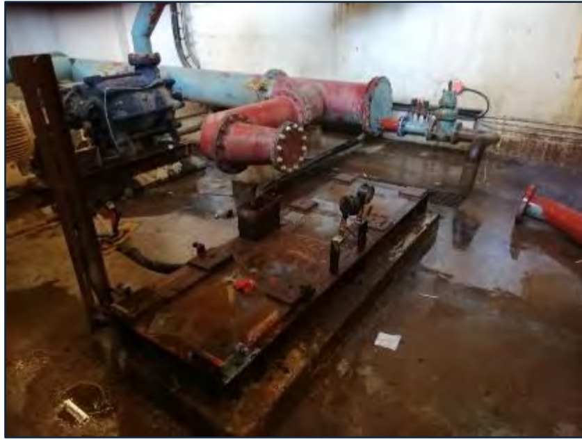
Figure 13.44 Petronella pump as of May 2019 (Umgeni Water 2019).
