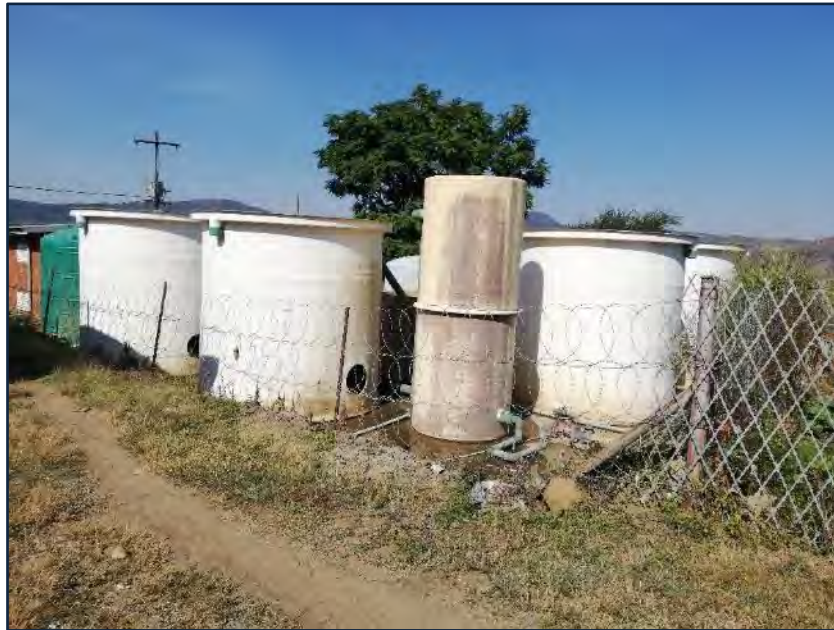
Figure 13.30 Tugela Estates WTP clarifiers (Umgeni Water 2019).
