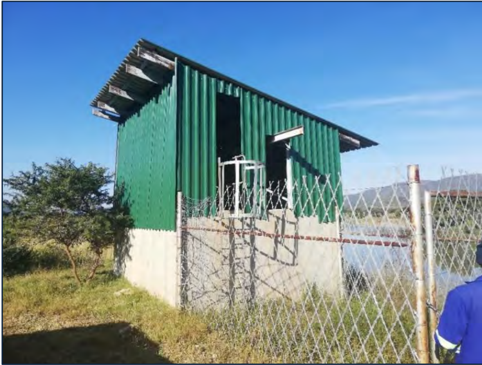
Figure 13.28 Tugela Estates Raw Water Pump Station (Umgeni Water 2019).
