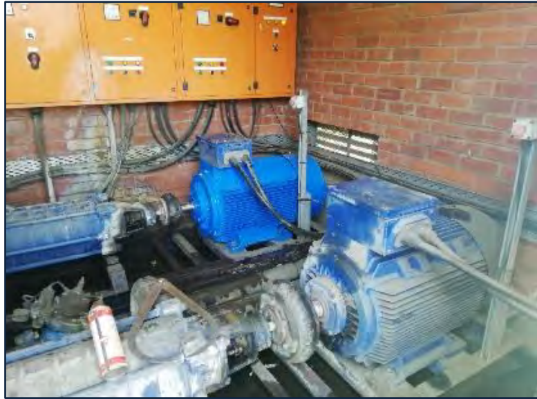
Figure 13.25 uMhlumayo Pump Station (Umgeni Water 2019).
