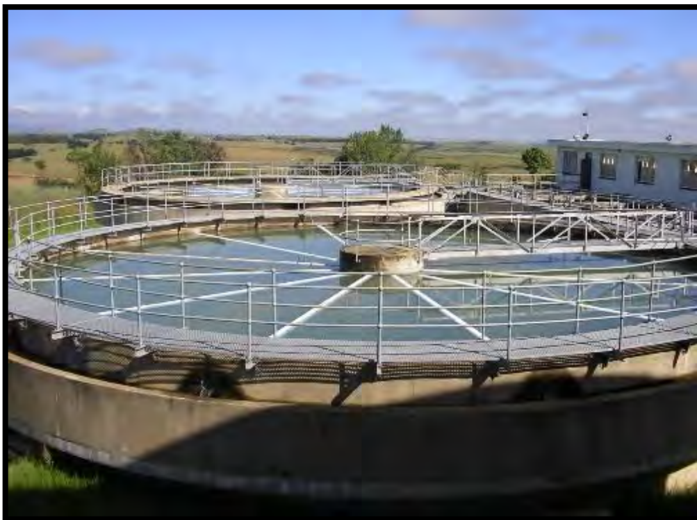
Figure 13.62 George Cross Water Treatment Plant (Bigen Africa, O & Manual, 2009)
