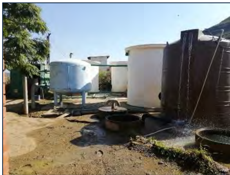
Figure 13.24 Tugela Estates Water Treatment Plant (Umgeni Water 2019).
