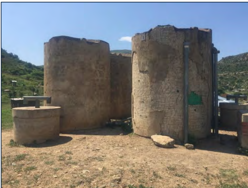
Figure 13.29 Tugela Estates Raw Water Holding Tanks (Umgeni Water 2019).
