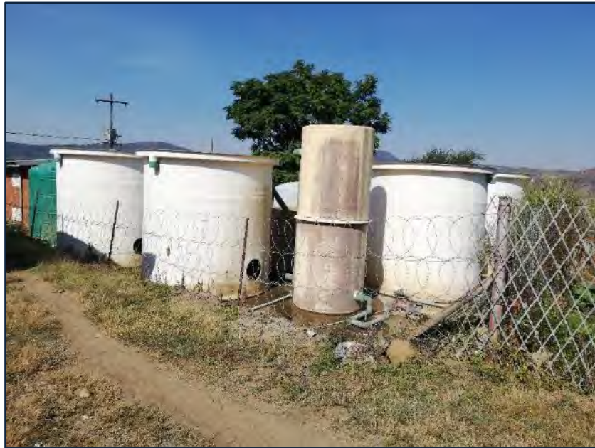
Figure 13.30 Tugela Estates WTP clarifiers (Umgeni Water 2019).
