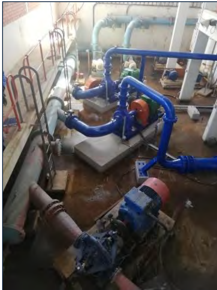
Figure 13.40 Olifantskop Clear Water Pump Station (Umgeni Water 2019).
