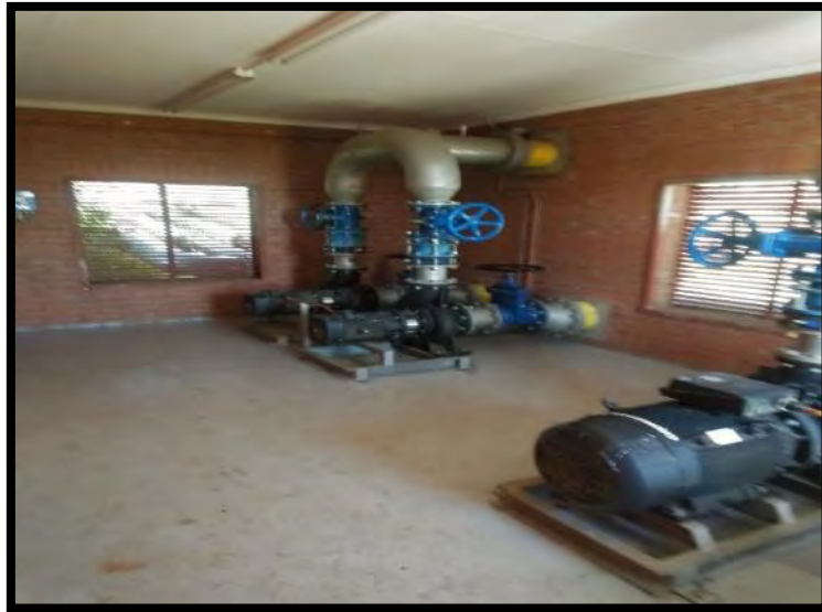
Figure 14.32 Durnacol Clear Water Pump Station (May 2020)
