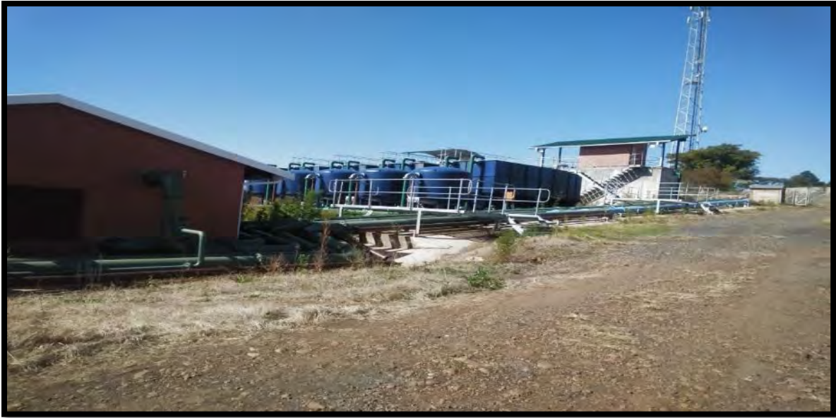
Figure 14.28 Photo of Durnacol Water Treatment Plant (May 2020).
