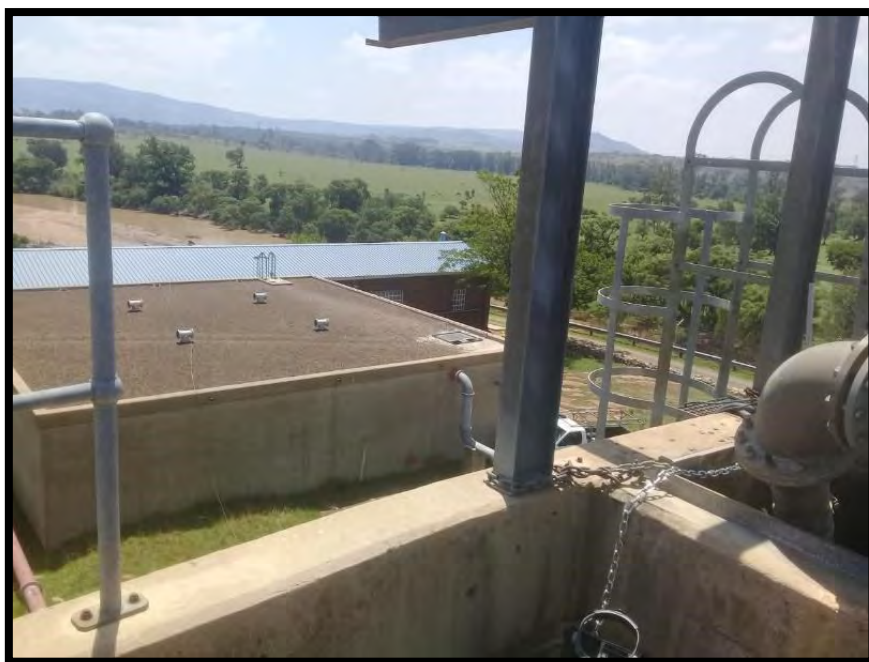
Figure 14.51 Photo of Vants Drift WTP (March 2020)
