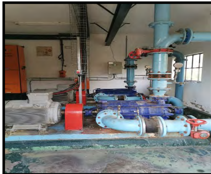
Figure 14.40 Utrecht Clear Water Pump Station
