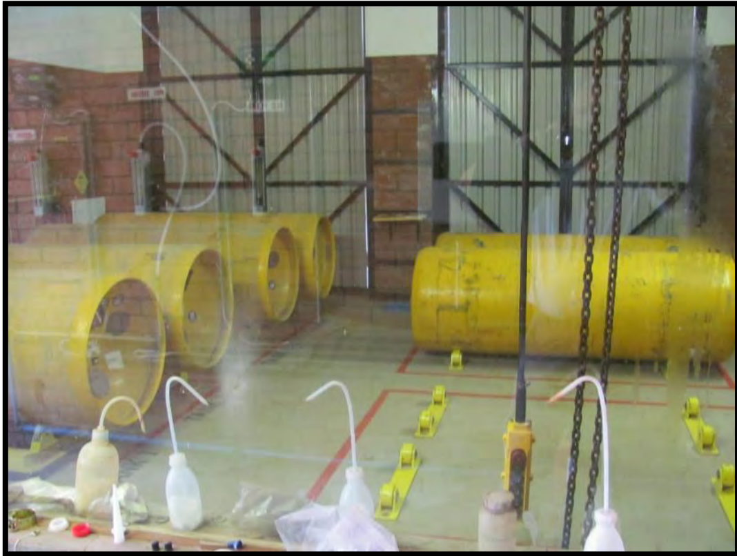
Figure 14.46 Photo of Chlorine Dosing Point at Biggarsberg WTP (July 2019).
