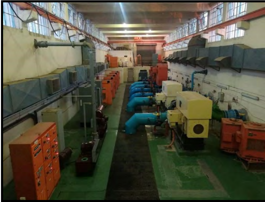
Figure 14.27 Photo of High Lift Pump Station at Ngagane WTP (May 2020)
