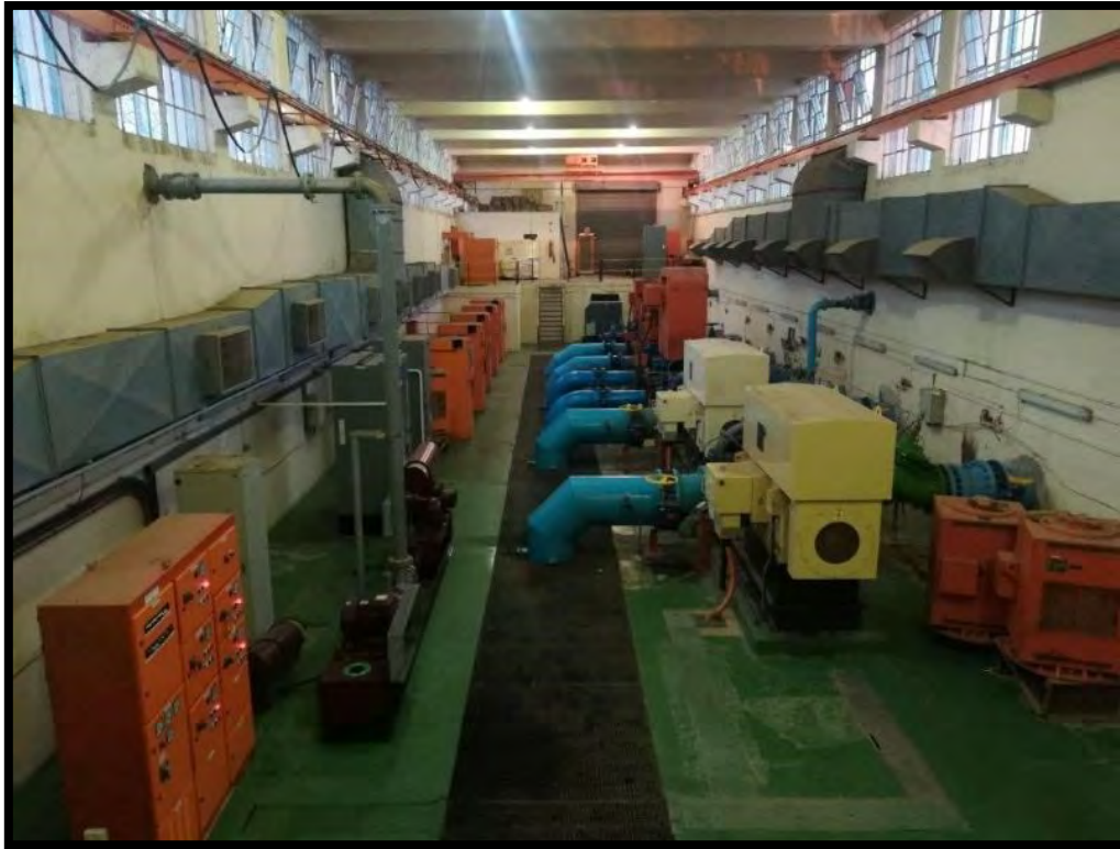
Figure 14.27 Photo of High Lift Pump Station at Ngagane WTP (May 2020)
